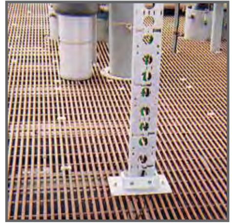
Offshore Oil & Gas Platform
