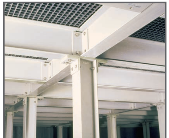
Advanced design and engineering of Dynaform structural shapes provide a lightweight, high strength support structure for this plating facility.
